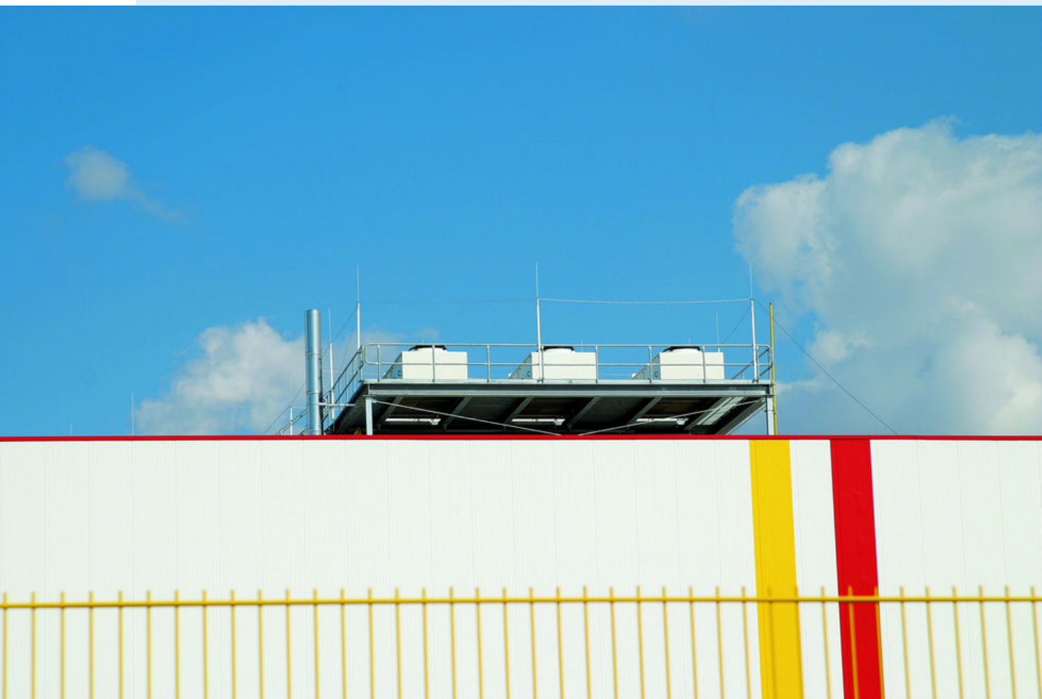
Güntner condensers equipped with lightning protection
