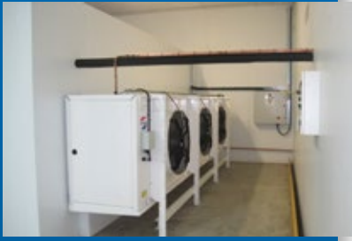
▲ The cooling equipment cools strawberries from 25 °C to 4 °C in the two-hour post-harvest period.
