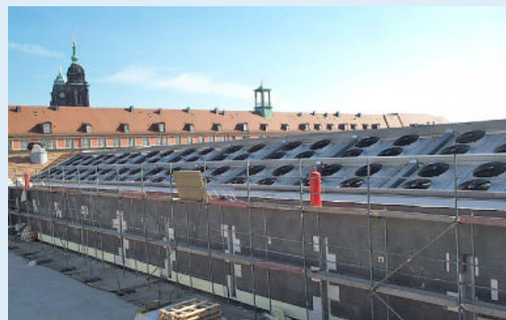
The 20 drycoolers installed in the pitched roof; in the background you can see the towers of Dresden's Kreuzkirche and the town hall
