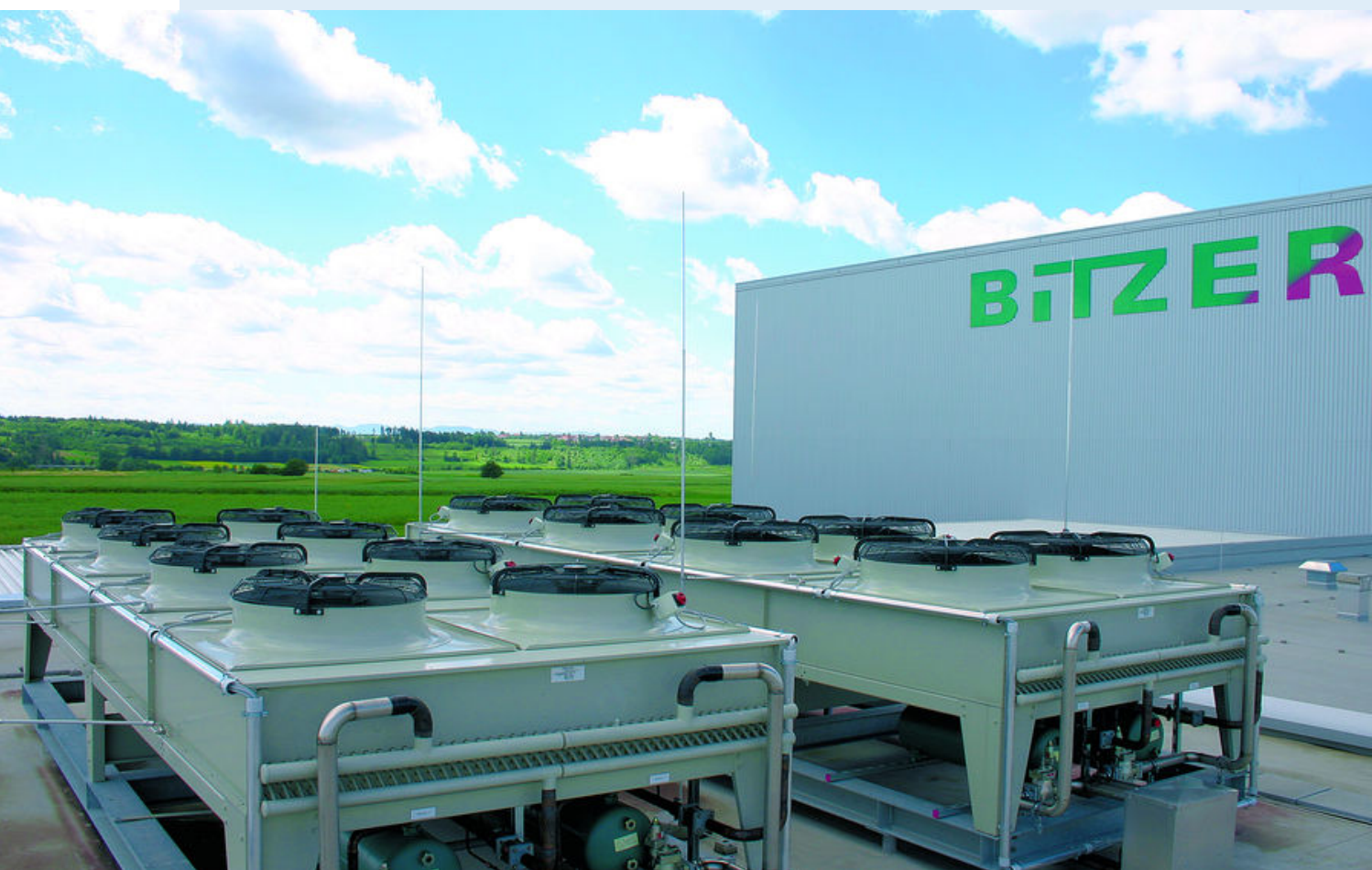
Air-cooled direct condensers from the GVH series made by Güntner. They are installed on the roof above the central cooling room of the new Bitzer factory in Rottenburg-Ergenzingen approximately 20 km south of Sindelfingen.
