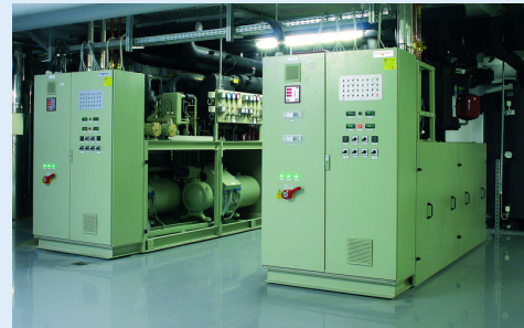
An exemplary central cooling system. Visitors are particularly impressed by the low noise levels of the Bitzer screw compressor.
