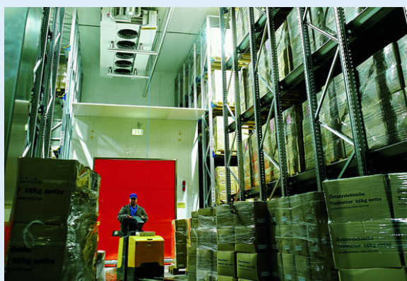
Maximum operative security with the Guntner NH 3 evaporators S-ADHN 066D/412 in a deep-freeze storage room
