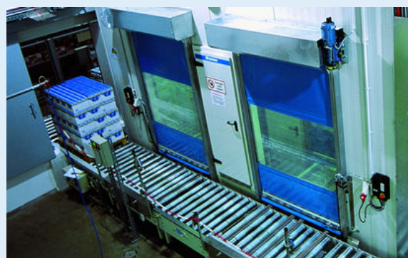
Tunnel cooler – chilling of yogurt from 20/25 °C down to 6 °C, 50 pallets per hour
