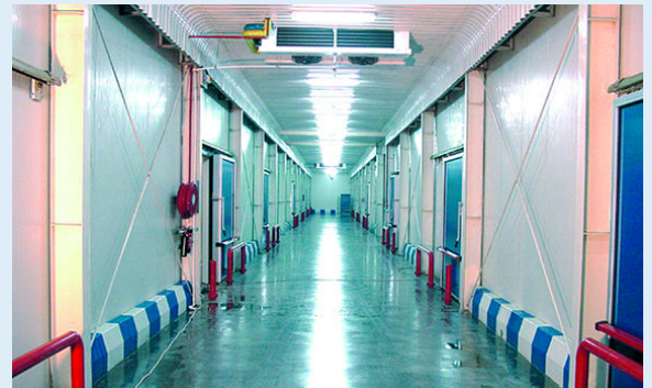
Connecting passages are cooled with S-GDS 051B/28 double coil evaporators
