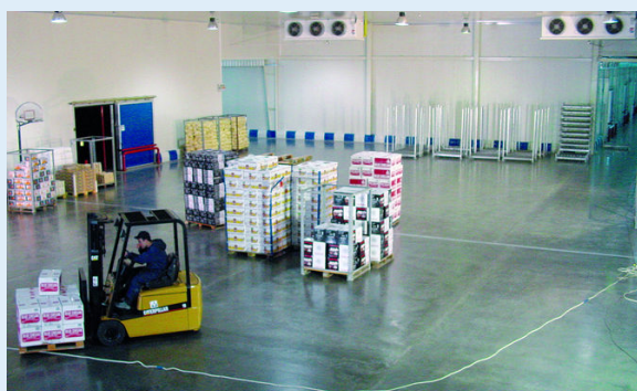
Two GHS 066D/38s lower the temperature in the large delivery and sorting hall to +10 °C
