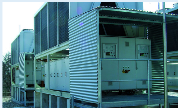
Front view of refrigeration machine
